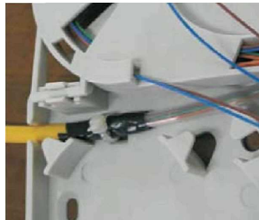
Pic12: put the pigtail through into the inlet port
