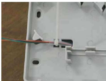
Pic6: dark-routing leads in box and fixes by nylon tie
