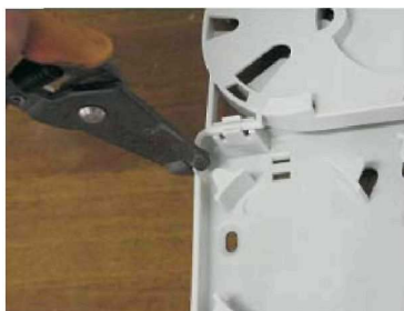
Pic7: right-routing leads in box entrance
